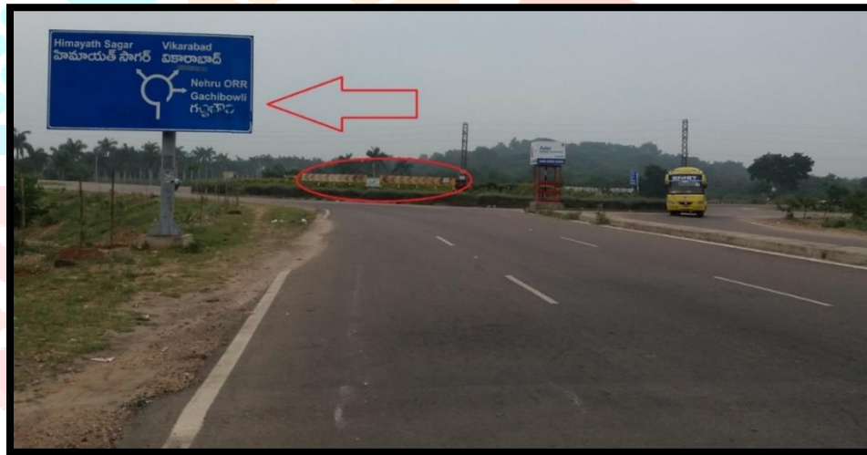
Fig 2 Retroreflective diversion boards faded
