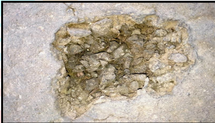
Fig. 3 Typical Pot Hole in Pavement before Repairing
