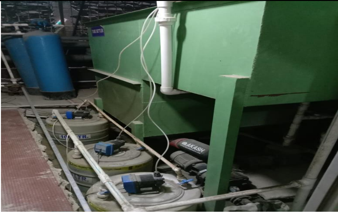
Fig. 3 ETP (effluent treatment plant) for waste water treatment process (WWTP)
