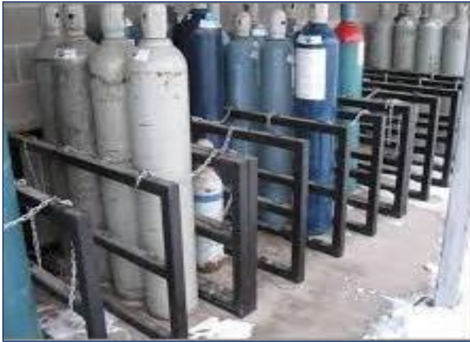
Figure-3: Representative compressed gas cylinder storage area showing cylinders stored upright in dedicated racks with chain restraints
