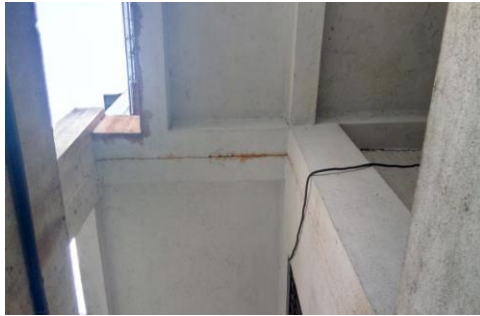
Fig. 3 - Horizontal cracks on beam
