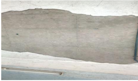
Fig. 1 - Spalling of paint
