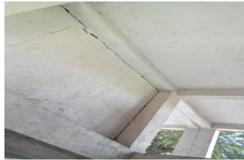
Fig. 4 - cracks on walls
