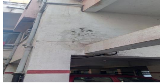
Fig. 2 - Seepage through walls
